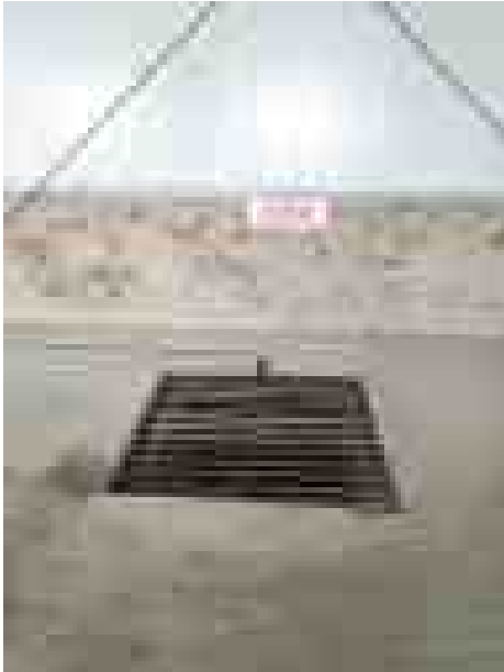
应急池及导流槽
